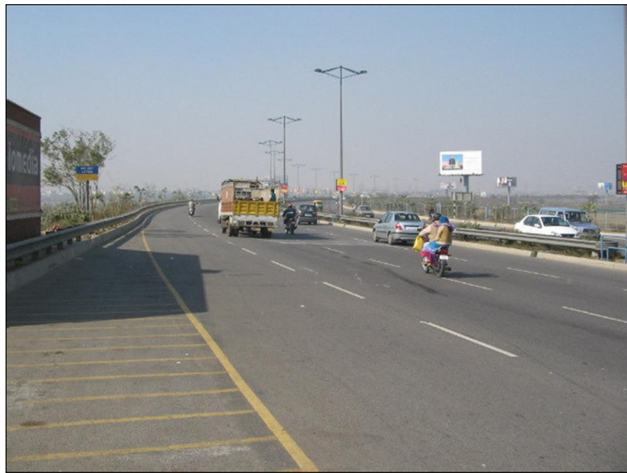
Figure 6 Existing Pavement Condition of DND Flyway
