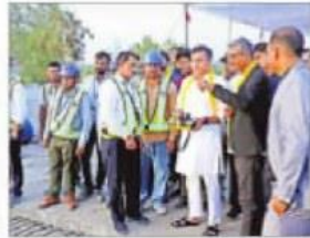
Work underway at the site (top); PWD Minister Parvesh Sahib Singh with the workers on Monday. EXPRESS
